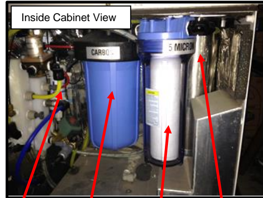
Capsule Filter .10" Carbon Block Filter 5 micron Filter 4" x 21" Membrane (inside stainless-steel housing)
