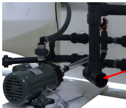
Bicarb Unit, Back View, Denoting Drain Connection
