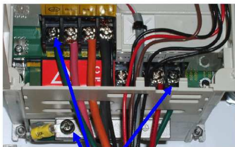
Old Model VFD Three ground wires
