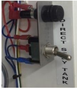
Switch Down – Tank Mode
